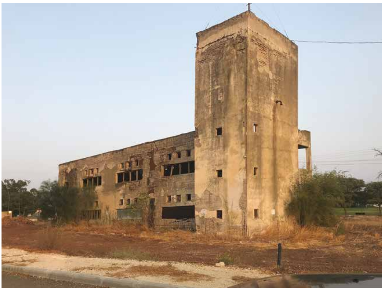
Illustration 1: Yosef Aharonovitz House in Moshav Beit Yosef, awaiting conservation. Photo: Irit Amit-Cohen
